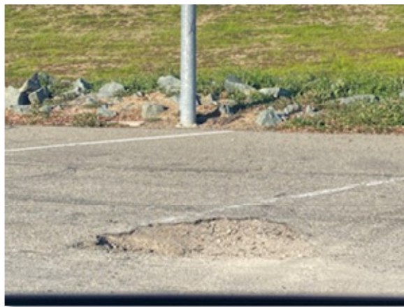
Parking lot with pothole.
