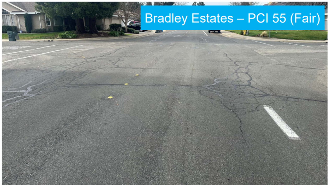
Example Photograph 1: Average condition of the road pavements of Yuba City today.
