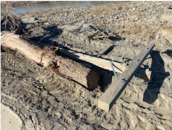
Downed telephone pole near the launch.
