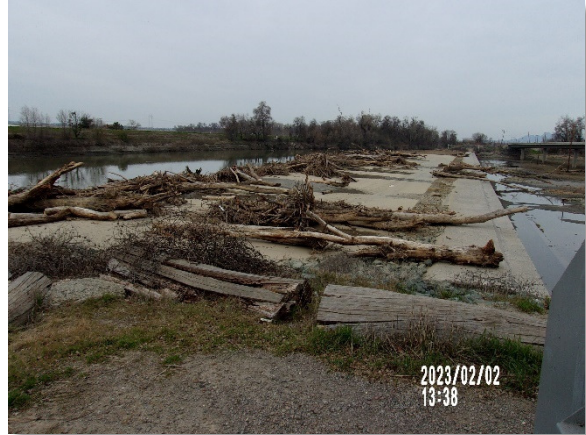
Debris from rising waters.
