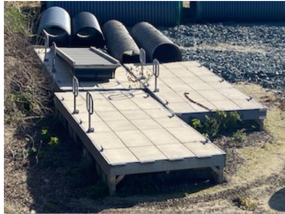
Floating dock not installed.
