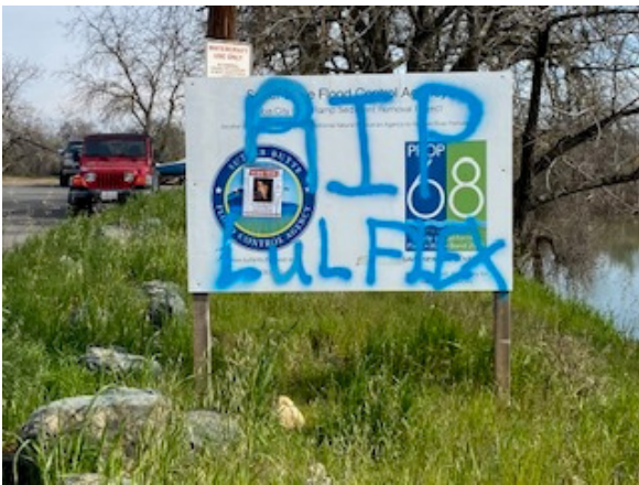
Poor signage conditions.
